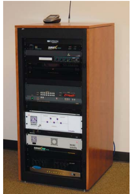
Close up of rack, containing the Audio Room Combining Matrix Mixer
